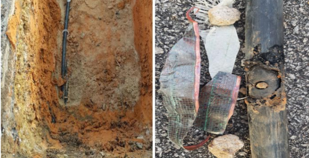
Fig. 17. Excavation at site found failure puncture on XLPE insulation.
