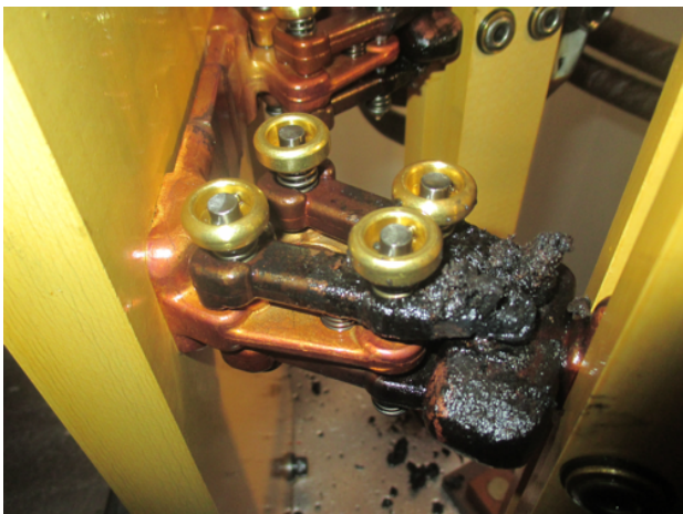
Fig. 15. Carbonization and overheating sign on changeover tap selector.
