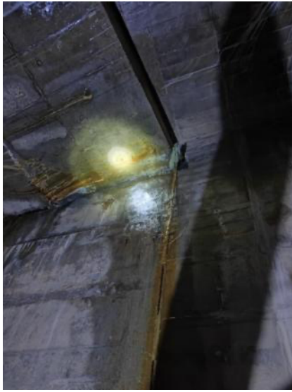
Fig. 1. Water Permeation in the Expansion Joints of Tunnels
