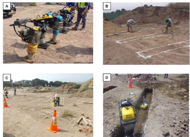
Fig. 2. Work site compaction activities: A) Rammer's set-up, B) Trench excavation process, C) Initial test with nuclear densometer, and D) Measuring soil density and moisture with the nuclear densometer.
