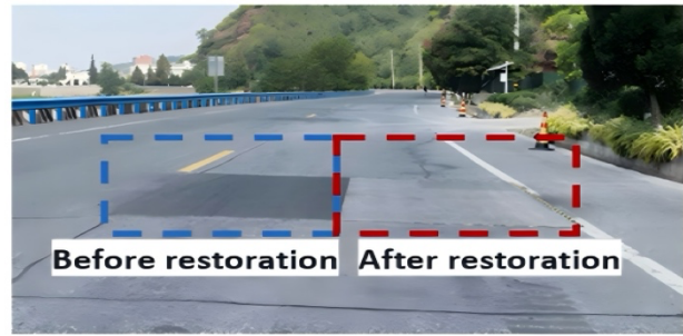
Fig. 11. Comparison before and after repair
