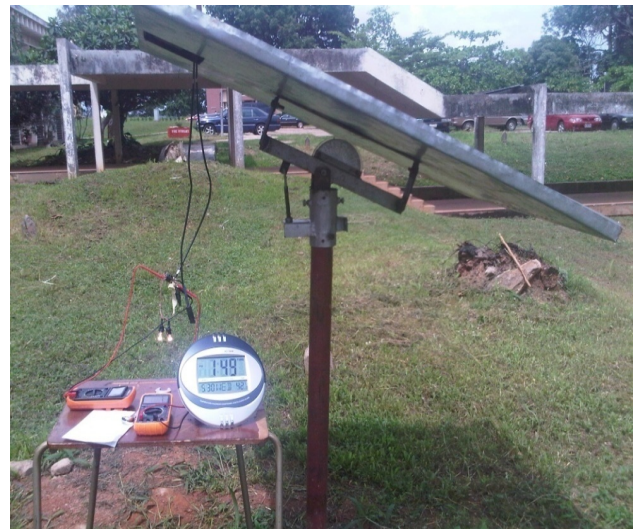
Fig. 1. Optimal tilt angle measurement for solar panel
